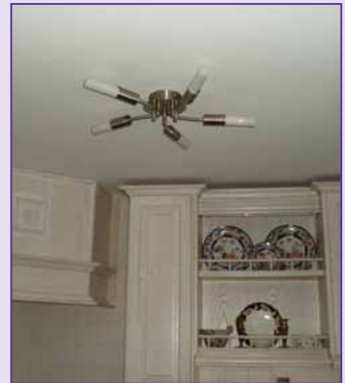
Compact fluorescent lamps reduce electricity demand for lighting to a quarter
